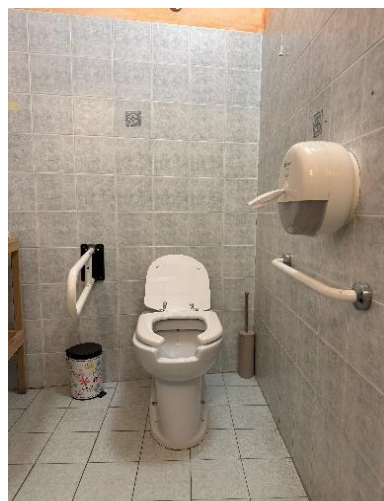
35 toilets with grab bars
